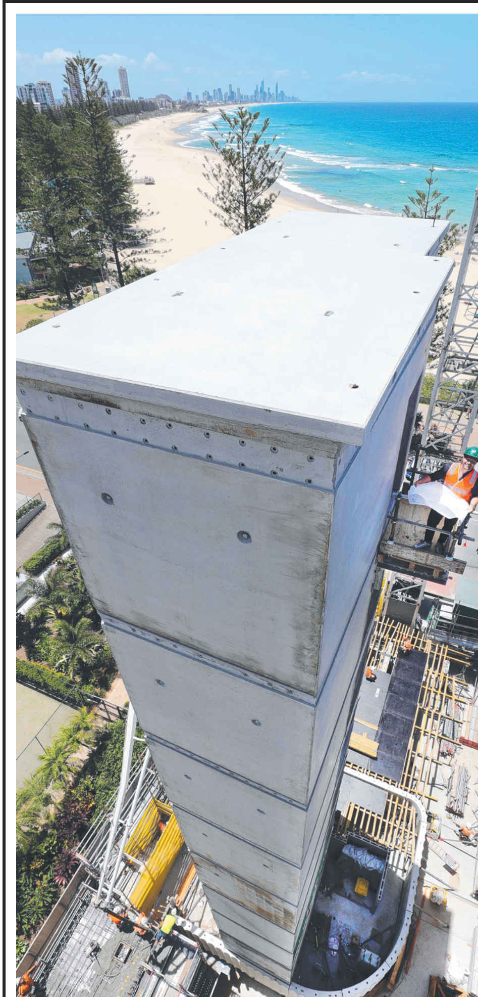
Developer David Calvisi at his Luna tower prefabricated stairwell and lift core on the Burleigh Heads beachfront. Picture: Glenn Hampson
